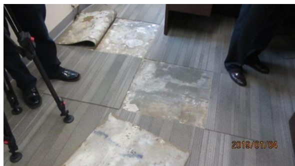
Photo #11 Carpet tiles removed adjacent to east wall in Investigations Room. Evidence of moisture and mold on backside of carpet tiles.
