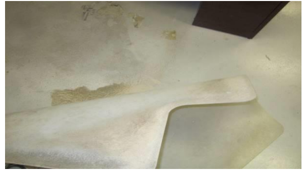
Photo #26 Visible mold and musty odor identified on underside of plastic floor mat on concrete floor in the Evidence Room (Tape Sample T12).
