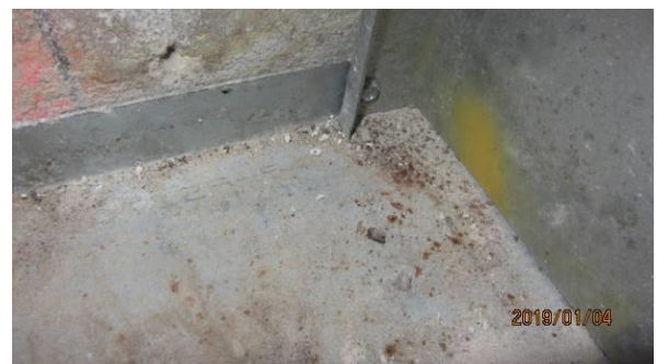
Photo #6 View of stud cavity in low wall cut at northeast quadrant. Some light corrosion noted in the track; no moisture evident.
