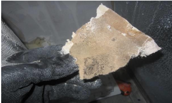
Photo #21 Visible mold on back side on drywall by Evidence Room freezer piping (Tape Sample T1).
