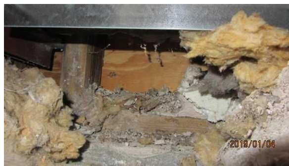
Photo #10 Cut at top of south wall, Training Room. Old wood dry and in good condition. Various types of debris on top of CMU, with possible bat droppings.
