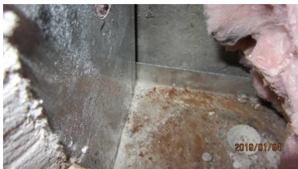
Photo #5 View of stud cavity in low wall cut at northwest quadrant. Some light corrosion noted in the track; no moisture evident.
