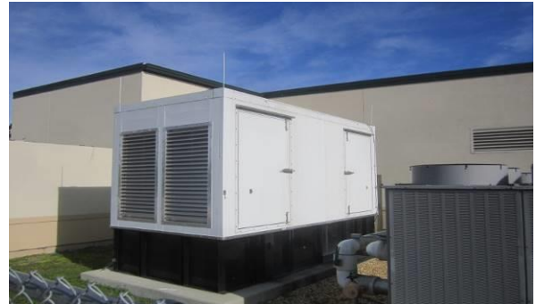
Photo #14 Emergency generator by make-up air intake along the southwest exterior.
