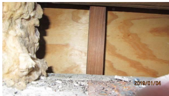
Photo #8 View of same cut. Some debris noted on top of the CMU wall; possibly rodent or bat droppings.
