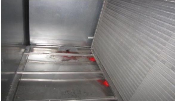
Photo #19 AHU condensate drain pan tablets.
