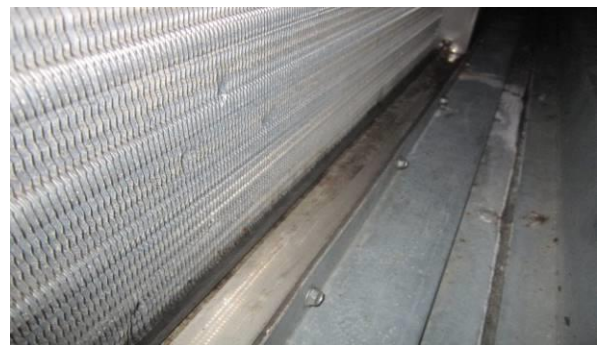
Photo #18 Visible mold at base of coils in AHU #1 serving the front lobby front lobby and northwest (Tape Sample T4).
