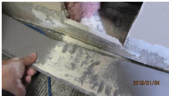
Photo #3 Low wall cut in Investigations Room. No moisture or evidence of mold in cavity or backside of vinyl base.
