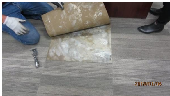
Photo #12 Carpet tile removed at location away from outside wall, same room. Evidence of moisture on slab.
