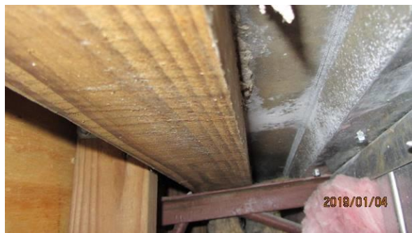
Photo #7 Cut at top of the wall in northwest quadrant. All wood blocking and framing dry and in good condition.
