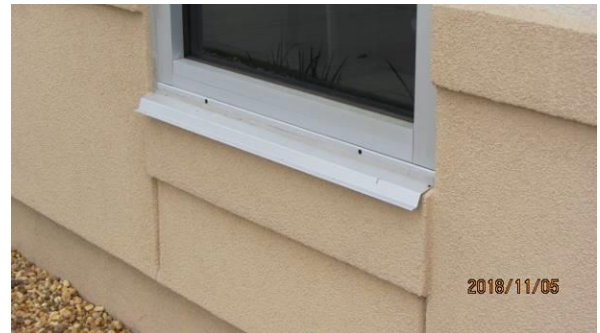
Photo #2 Typical window sill with pan flashing and weep holes in the extrusion above the pan.
