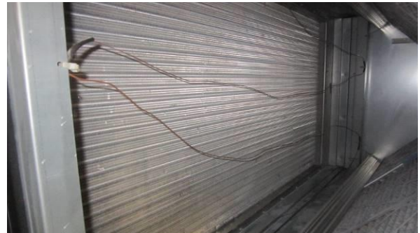
Photo #16 Coils in AHU #2.
