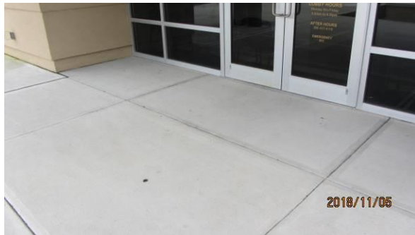
Photo #1 Paving at front entrance. Flush with floor level and basically flat without slope to drain.
