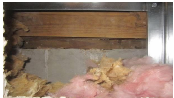
Photo #24 Older wood with high mold counts on top of concrete block perimeter wall in the Evidence Room (Tape Sample T11).
