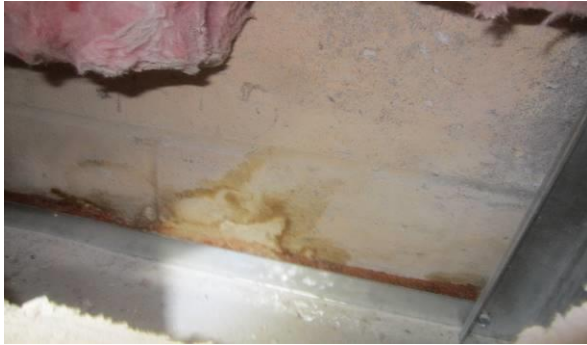
Photo #25 Water stain on Evidence Room block wall.
