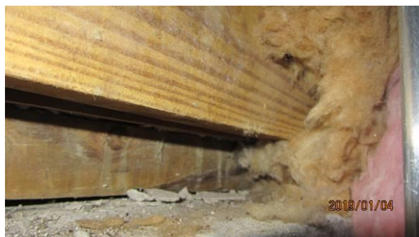
Photo #9 Cut at top of wall in Main Evidence room. Old insulation (yellow) and new insulation (pink) are noted. Recessed wood is original; dry, good condition.
