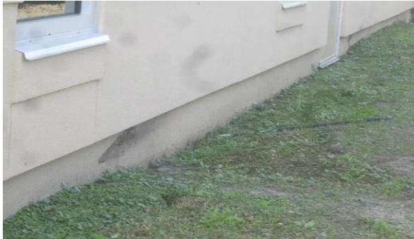
Photo #13 Low drainage areas along east exterior.
