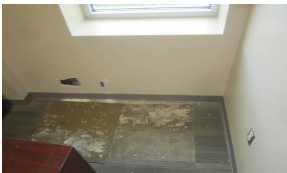
Photo #23 Visible mold and musty odor below carpet square in Investigations Room 129 (Tape Sample T10).
