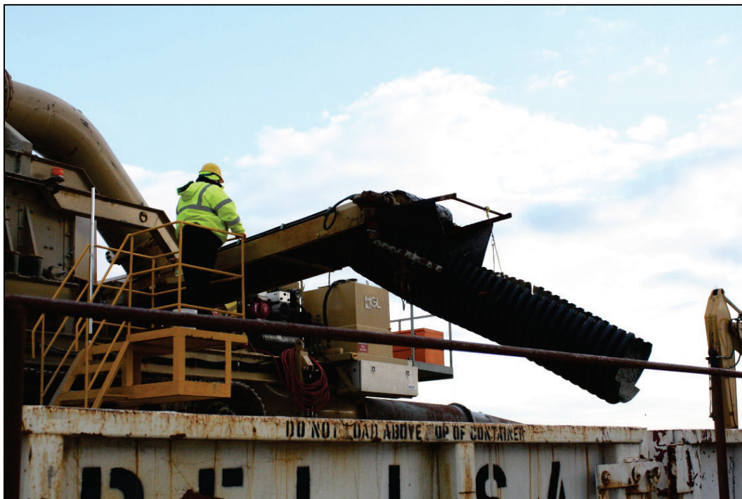
Figure 19. FRS unit modified for use in a beach nourishment project in Deal, NJ, that involved MEC.
