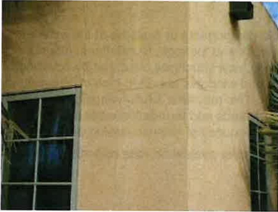
Photo 11-1 STUCCO CRACKS SEVERAL LOCATIONS
