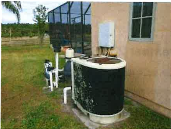
Photo 2-1 POOL ELECTRIC HEATER NOT WORKING
