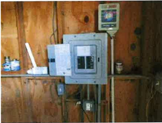
Photo 22-7 SHED SUB PANEL
