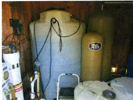
Photo 26-4 WATER HOLDING TANK
