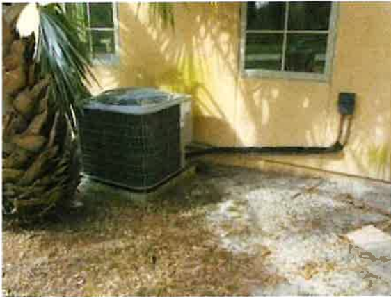
Photo 30-1 HOUSE COMPRESSOR 4 TON INSTALLED IN 2021 REPIPED THROUGH GARAGE TO AIR HANDLER NO ATTIC ACCESS
