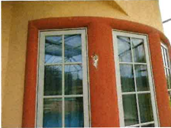
Photo 35-1 METAL FRAME WINDOWS /CASEMENTS. WINDOW SEALS DAMAGED IN LOWER CORNERS . SUSPECT WATER INTRUSION INTO WALLS. HOUSE INSULATED WITH CLOSE CELLED MATERIAL THE REASON FOR STUCCO REPAIRS. WINDOW TRIM MINOR DAMAGE TO STUCCO
