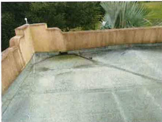
Photo 15-1 ROOF DECK A FEW AIR POCKETS
