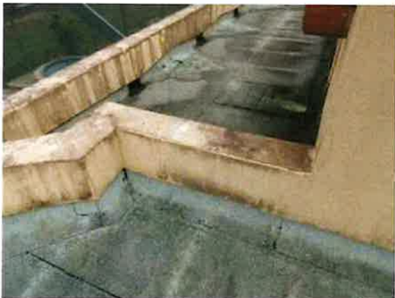
Photo 15-7 ROOF CAP AIR BUBBLES
