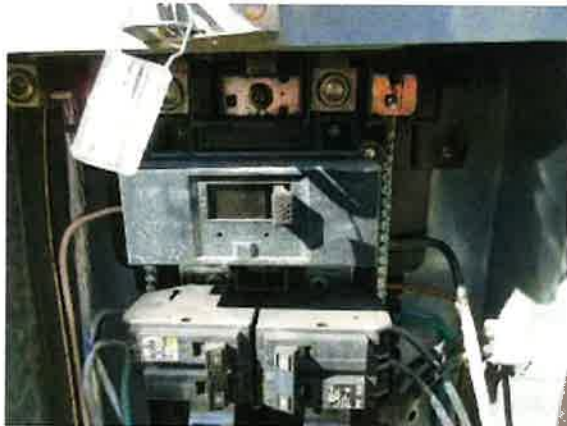
Photo 22-3 200A MAIN BREAKER
