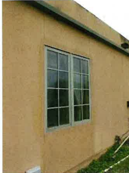
Photo 35-2 WINDOW METAL CASEMENT STUCCO REPAIR CLOSED CELL INSULATION WATER INTRUSION
