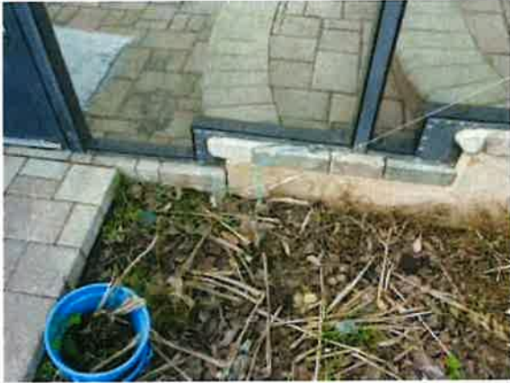
Photo 2-3 CABELS FOR POOL SCREEN NEED TO TIGHTENED
