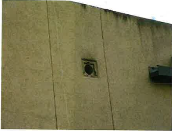
Photo 12-7 EXHAUST VENT DAMPER MISSING
