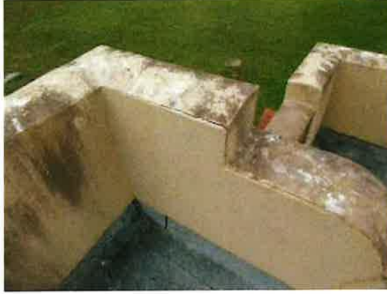
Photo 15-10 WALL /CAP CRACK 1/8 OPEN
