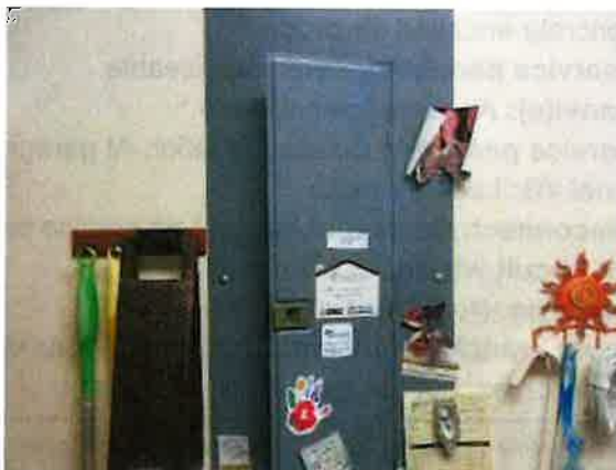
Photo 22-4 SUB PANEL IN LAUNDRY ROOM
