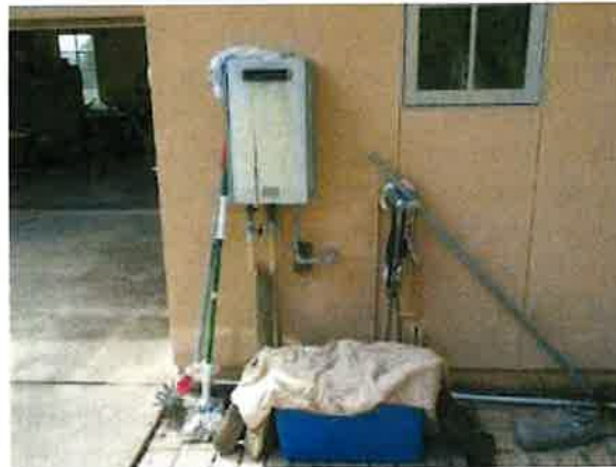
Photo 28-2 WHOLE HOUSE WATER HEATER
