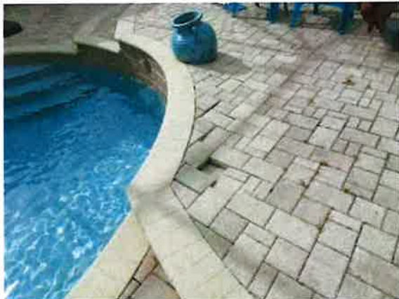
Photo 2-7 POOL DECK FAILURE
