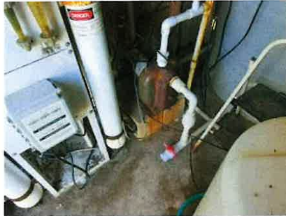
Photo 26-2 WATER PUMP FROM HOLDING TANK FOR HOUSE WATER
