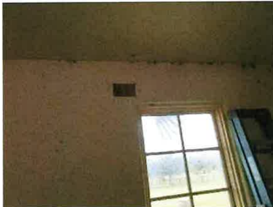
Photo 17-2 SHEET ROCK CUT OUT
