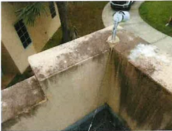
Photo 15-11 CAMERA ON WALL CAP SCREWED DOWN
