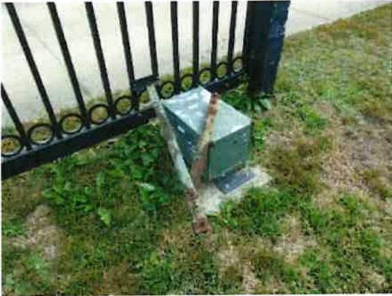
Photo 3-3 GATE CONTROL BOX
