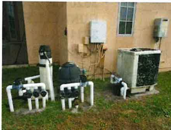
Photo 2-2 POOL EQUIPMENT RASZL POOL REPORT ADDRESS THIS
