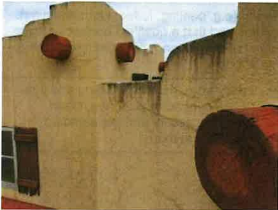
Photo 11-5 WALL CRACKS IN STUCCO
