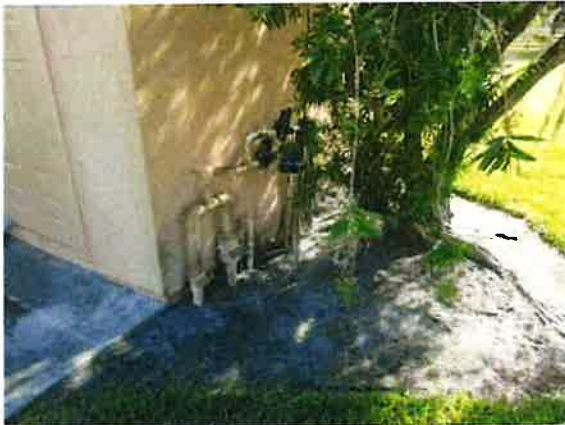
Photo 4-1 IRR SYSTEM NOT PART OF INSPECTION
