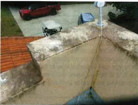
Photo 15-5 WALL /CAP CRACK JOINT
