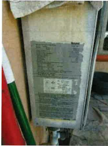
Photo 26-6 GAS WATER HEATER DATA
