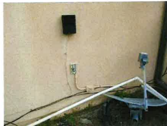
Photo 12-6 EXTERIOR OUTLET BOX MISSING COVER
