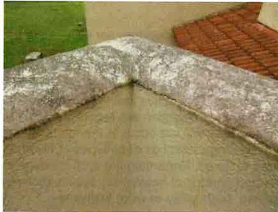
Photo 15-4 CAP WALL JOINT/ CRACK LINE
