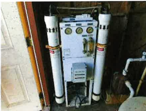
Photo 26-3 REVERSE OSMO WATER TREATMENT SYSTEM ,DUMPS EXCESS WATER TO EXTERIOR OF SHED . WATER COLLECTING AND PONDING
