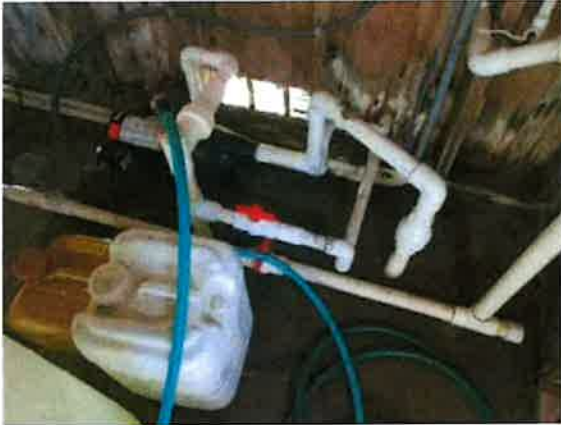
Photo 26-1 MAIN WATER SHUT OFF IN SHED
