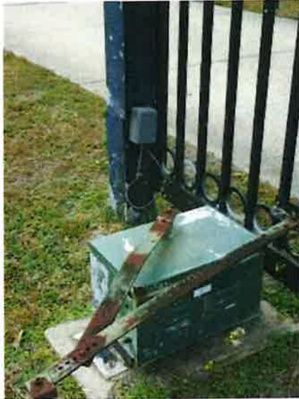
Photo 3-4 GATE CONTROL BOX
