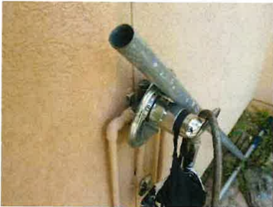
Photo 27-1 EXT SHOWER CAPPED OF TO SHOWER HEAD
