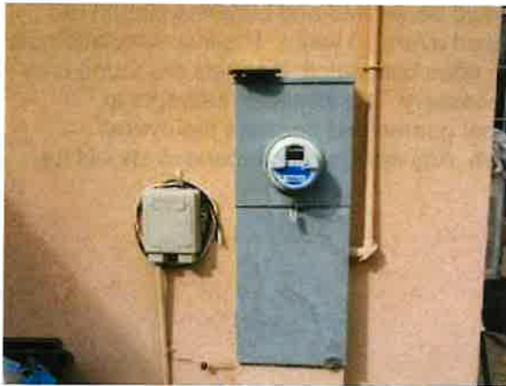
Photo 22-1 MAIN 200 AMP ELECTRIC PANEL RIGHT SIDE OF GARAGE
