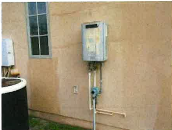
Photo 28-1 POOL GAS HEATER
