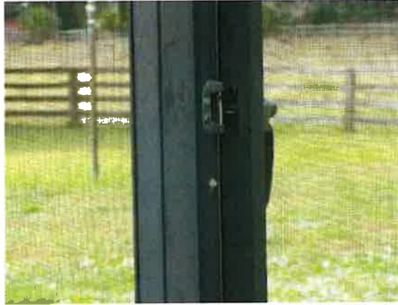
Photo 2-6 SCREEN DOOR LATCH BROKEN
