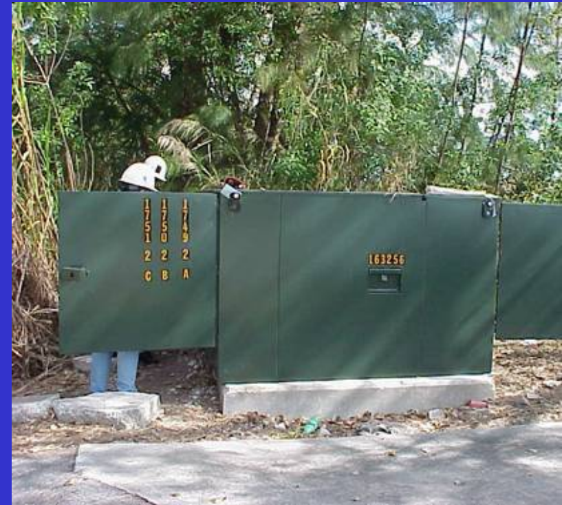
Pad Mounted Switch Cabinet
