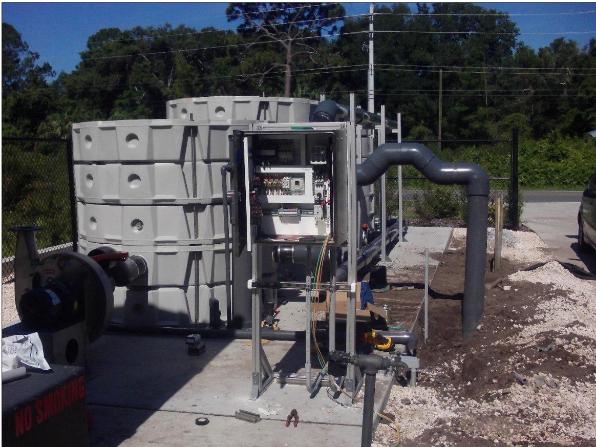
Old Kings Road Odor Control Units
