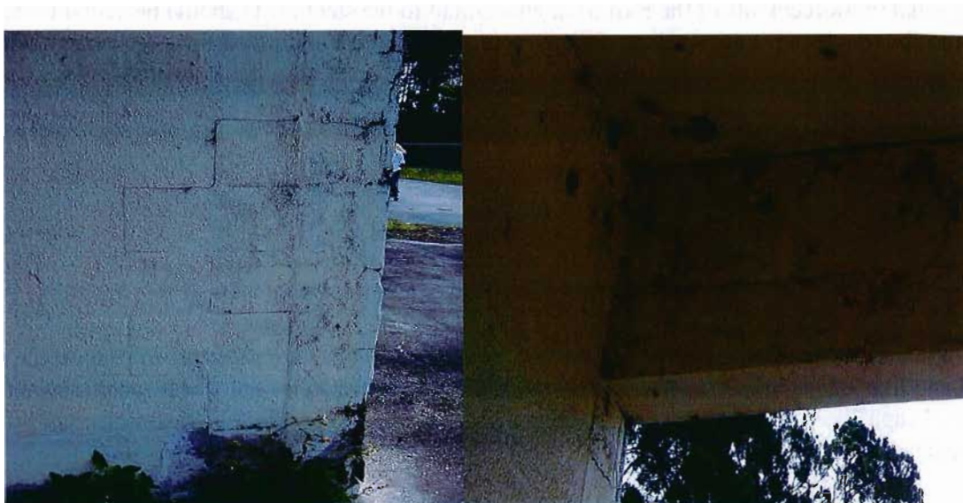
Settlement Cracking in CMU Wall and Concrete Beam
