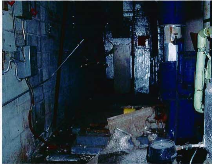
Missing Chilled Water Pumps
