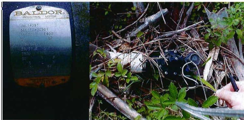
Irrigation Pump and Typical Zone Control Valve
