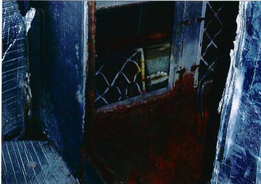
Photo 1 – AHU Interior in Mechanical Room
