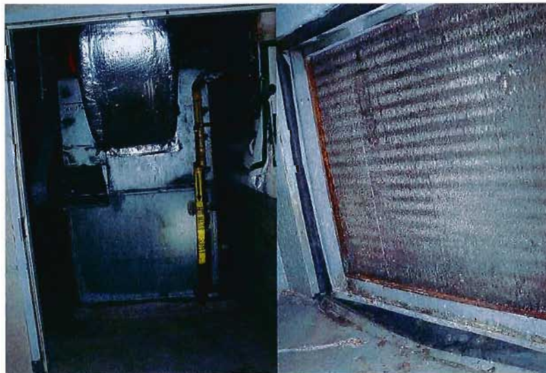
Typical AHU and Coil
