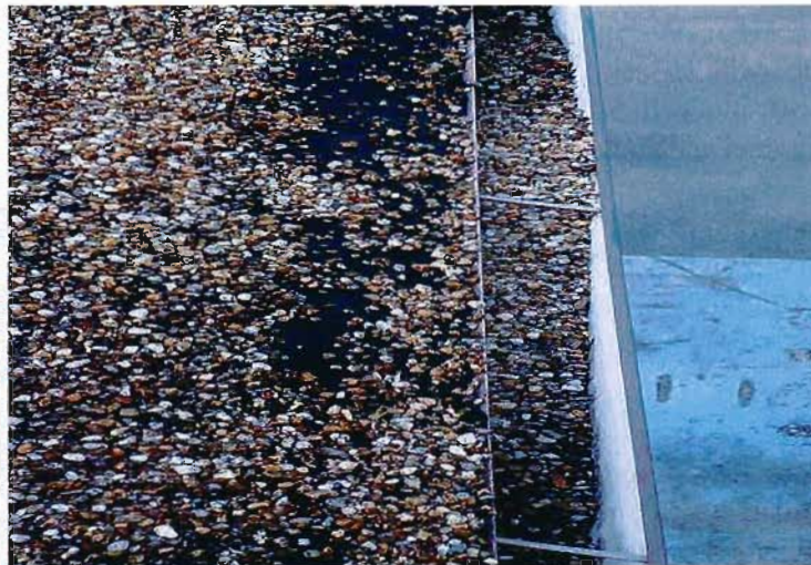
Gutter Filled with Gravel from Roof Membrane
