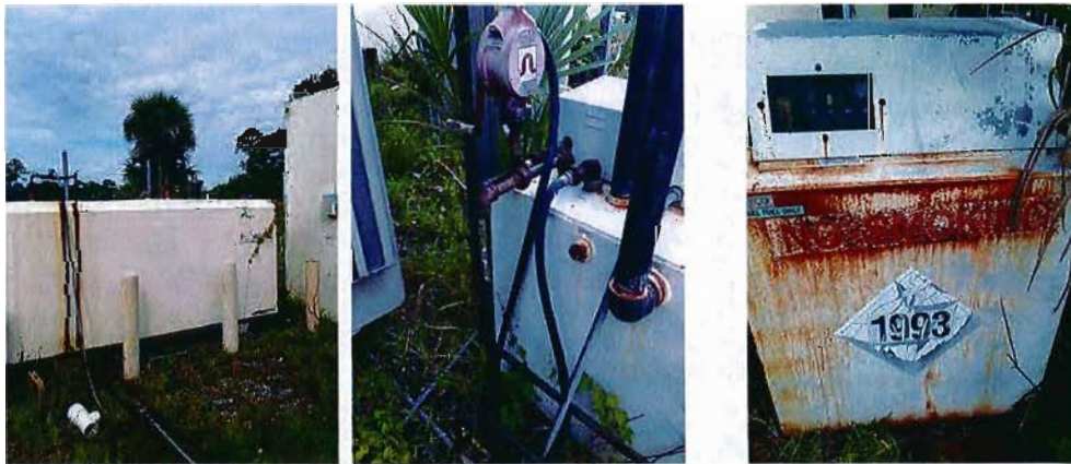
Generator Fuel Tank and Pump
