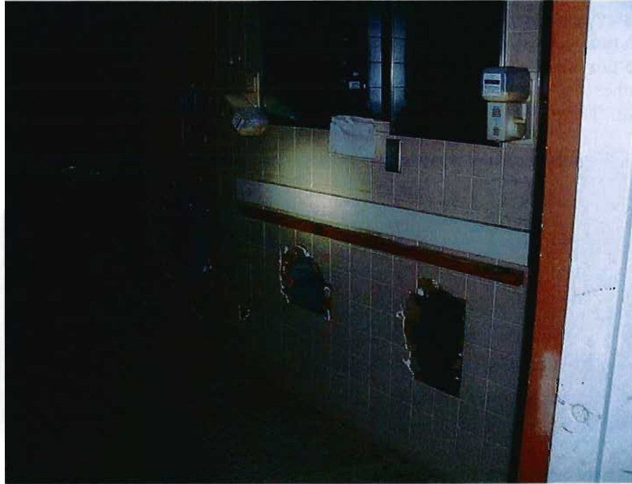
Typical Plumbing Conditions
