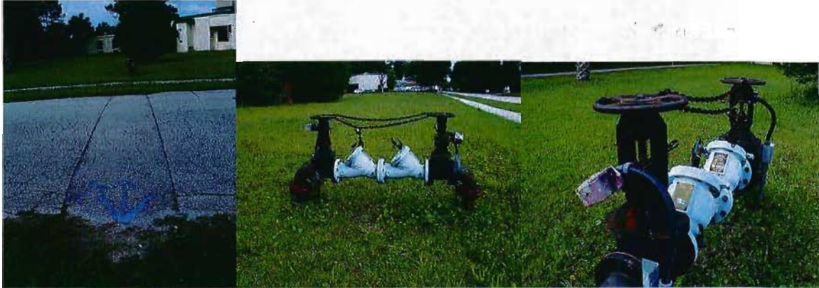
Potable Water Entrance
