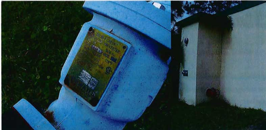
Potable Water Check Valve (left) FDC and Entrance (right)
