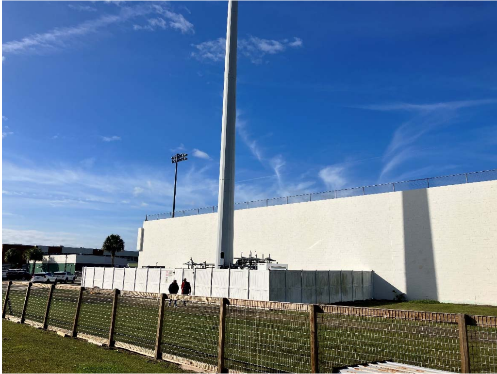
Figure 6: Site Photo – Equipment Compound Northeast facing Southwest
