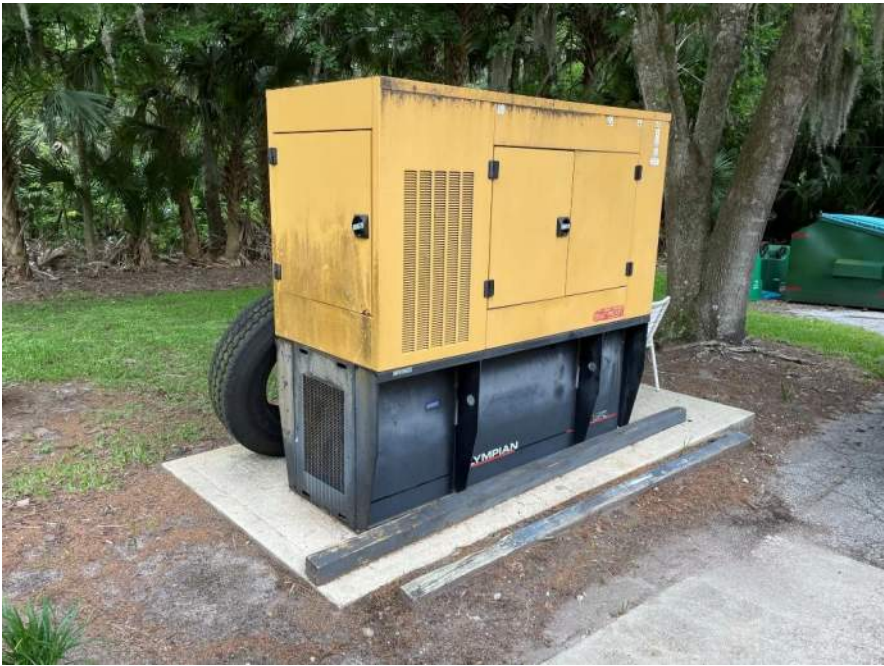
IMG_4323: Generator and diesel fuel tank
