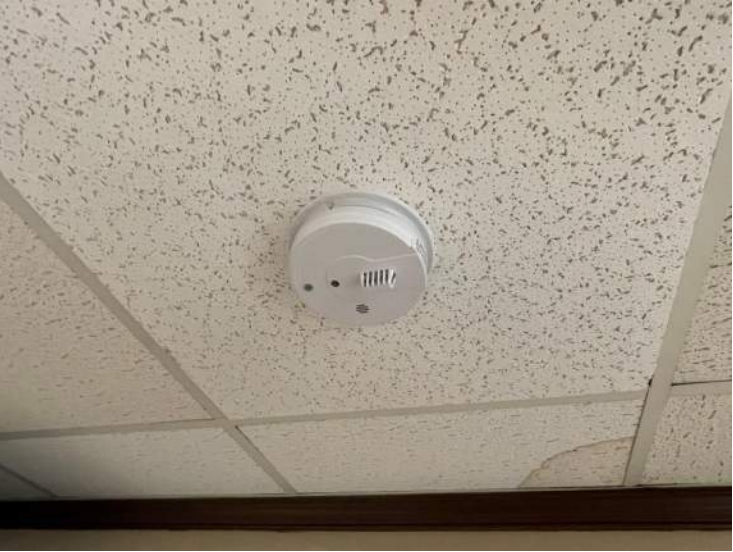
IMG_4380: Stand alone smoke detector in Dayroom
