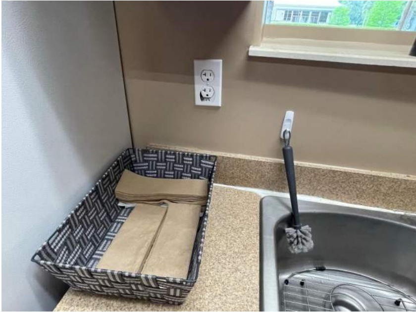
IMG_4383: Cracked/damaged faceplate
