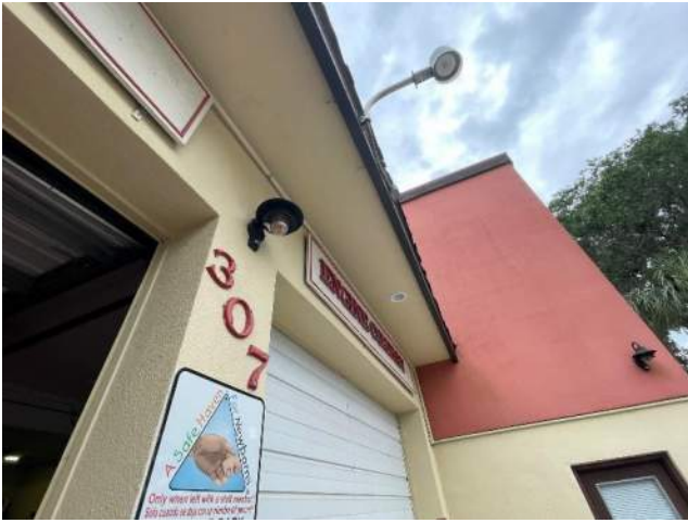
IMG_4332: Building mounted lights of various types
