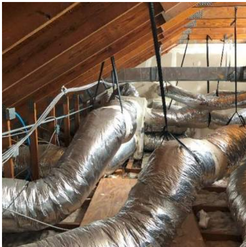
IMG_7885: Spaghetti flex duct distribution
