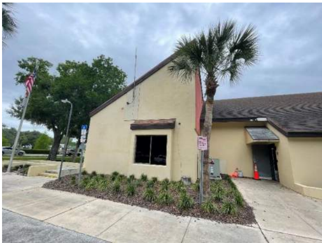
IMG_4336: Steel pole mounted light
