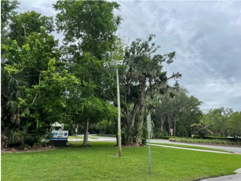
IMG_4350: Wood pole mounted lights
