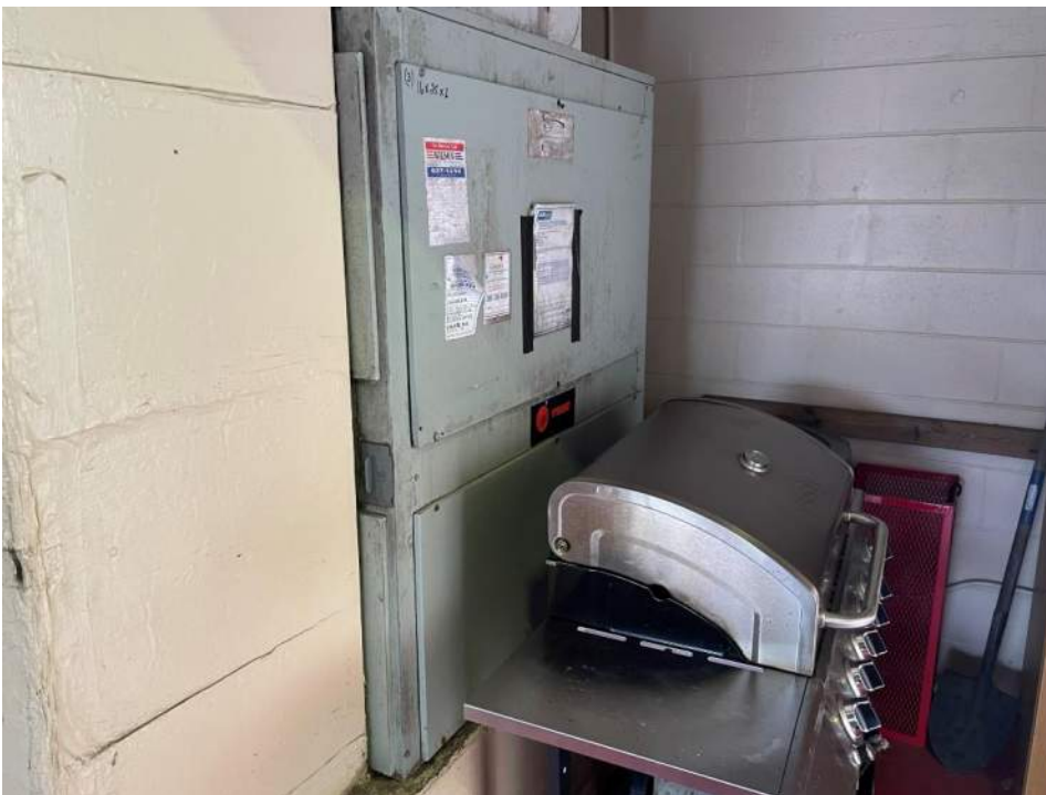
IMG_4310: AHU showing visible mildew growth on the housing
