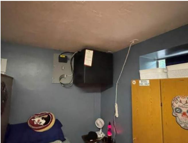
IMG_4432: Communication rack located above sleeping bunk
