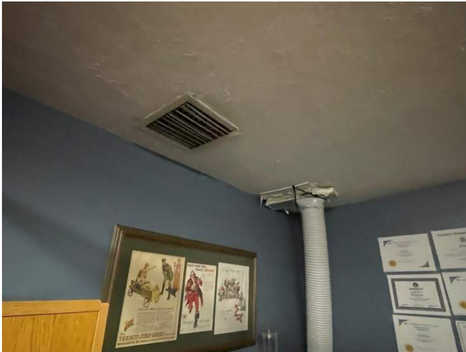
IMG_4441: Heat discharge from portable unit extending through ceiling into attic
