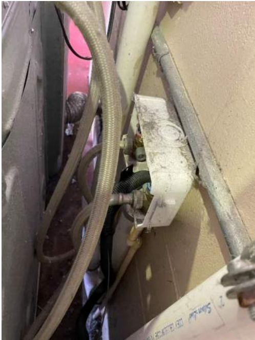
IMG_4460: Wash Box is in poor condition
