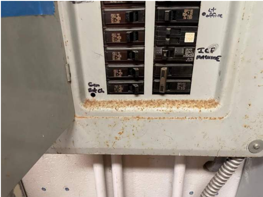
IMG_4277: Rusting conditions on 45 year old panels
