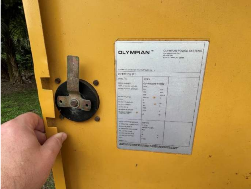
IMG_4416: Generator nameplate
