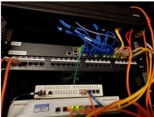
IMG_4437: Rack interior with patch panel and cabling
