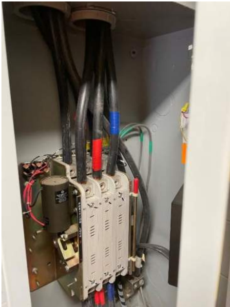
IMG_4281: ATS interior
