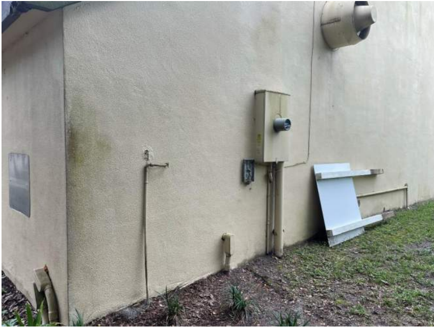
IMG_0766: Exhaust louver on east wall and make-up air louvers in clearstory window
