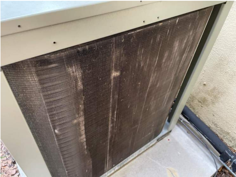
IMG_4317: Corrosion visible on condensing unit coil
