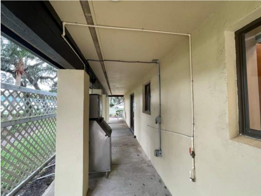
IMG_4342: Unprotected Domestic water piping for Icemaker subject to mechanical damage
