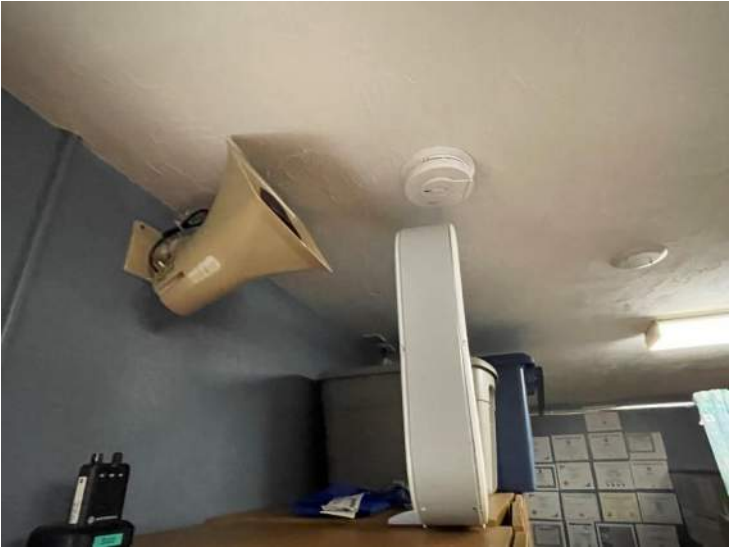
IMG_4422: Stand alone smoke detector in bunk room
