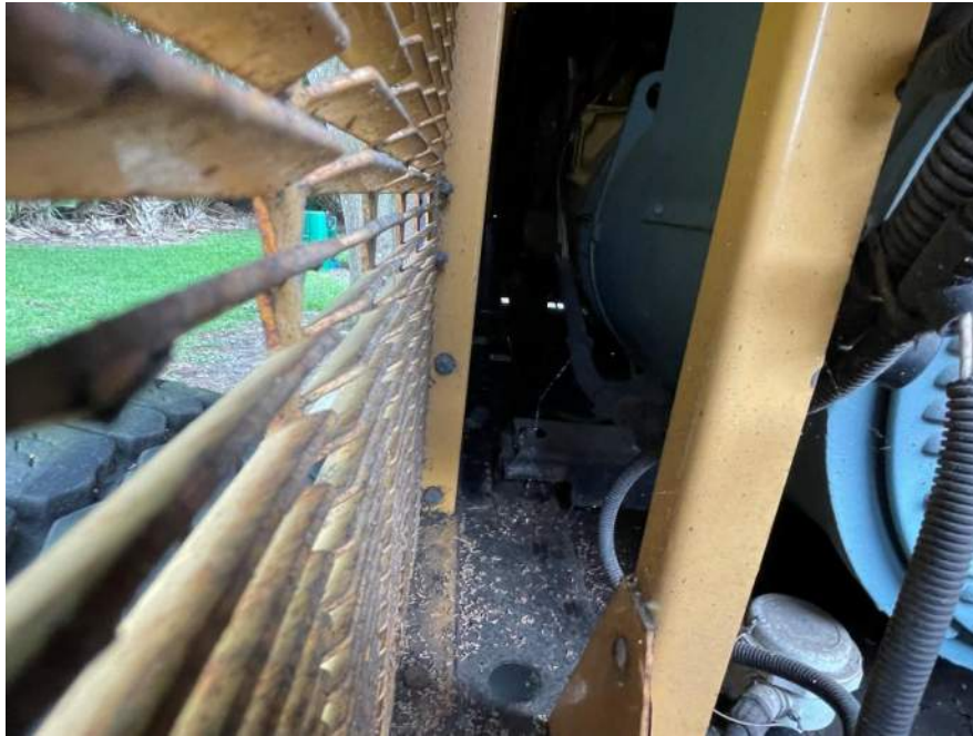
IMG_4420: Generator interior
