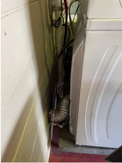
IMG_4460: Laundry Wash box in poor condition
