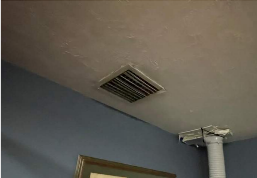
IMG_4441: Damaged supply diffuser
