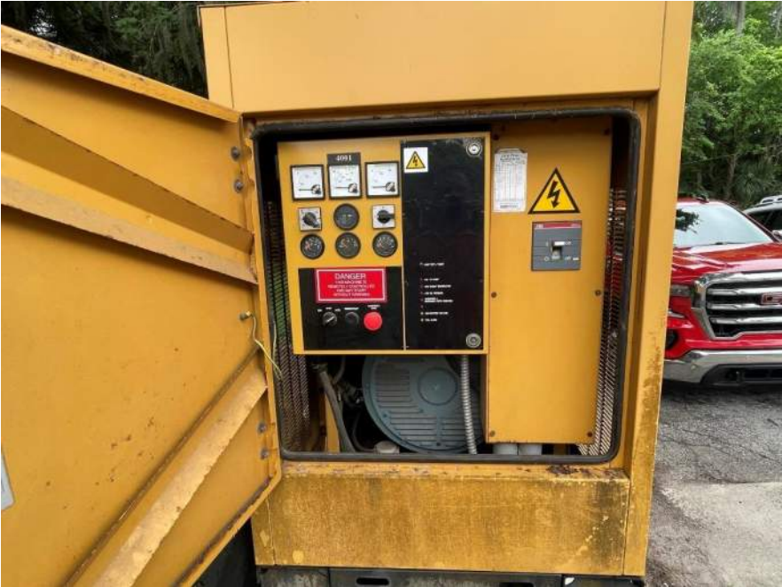
IMG_4418: Generator control panel
