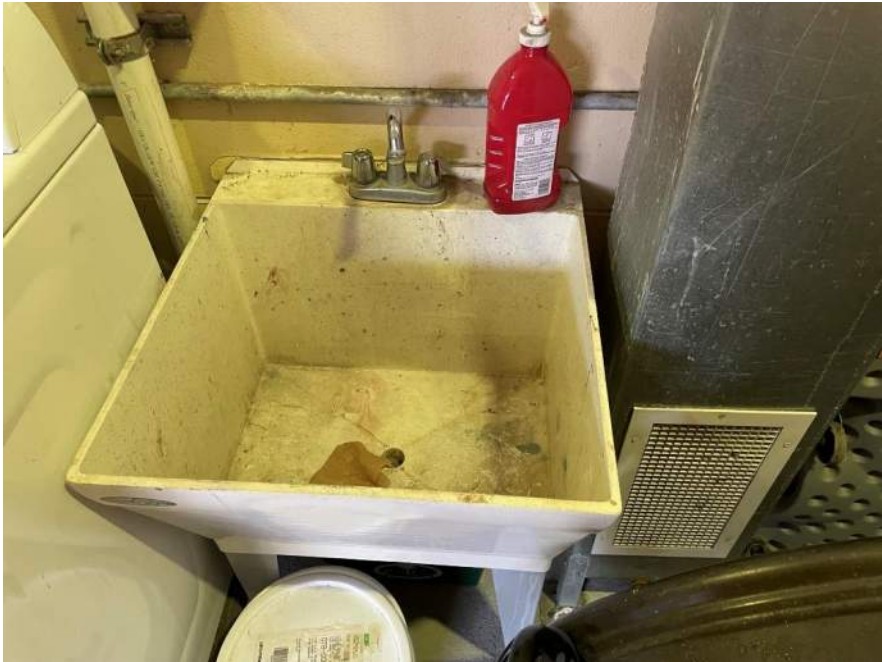
IMG_4304: Laundry Tub (Service sink) rusted and stained.
