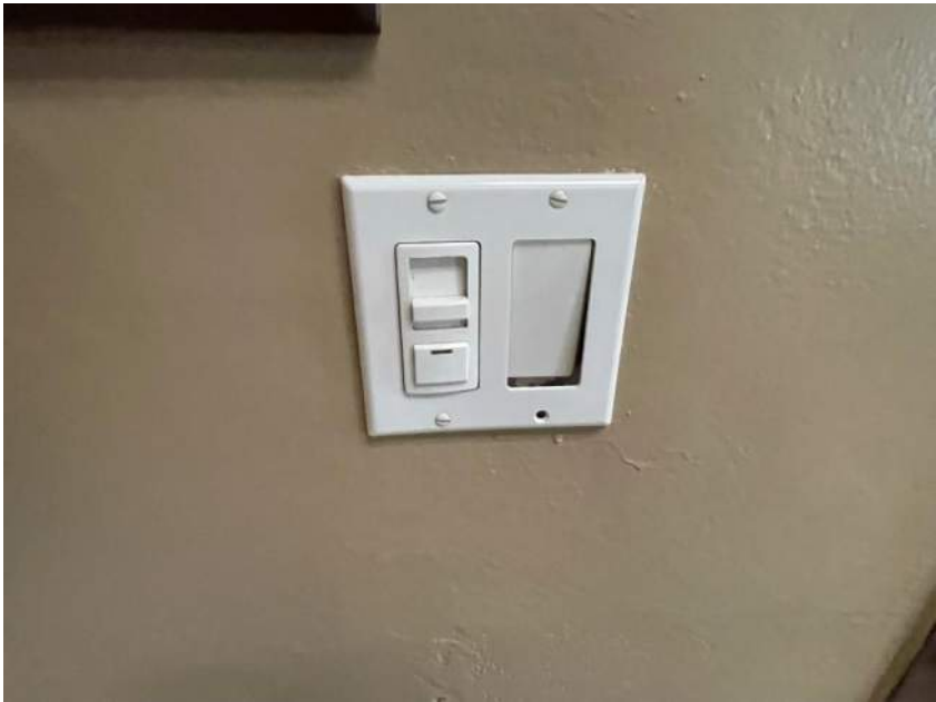
IMG_4403: Cracked/damaged faceplate
