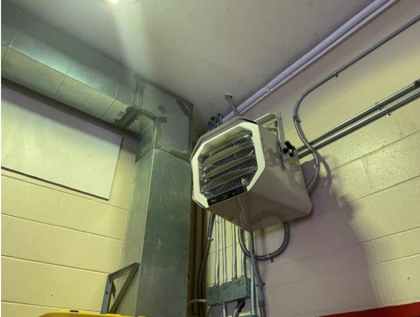
IMG_4292: Electric unit heater in the apparatus bay
