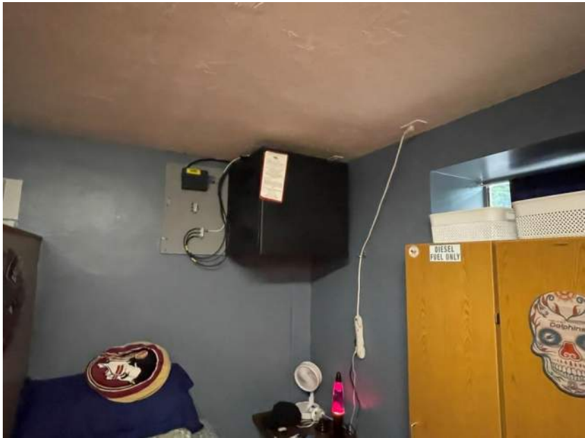
IMG_4432: Not enough outlets in bunks
