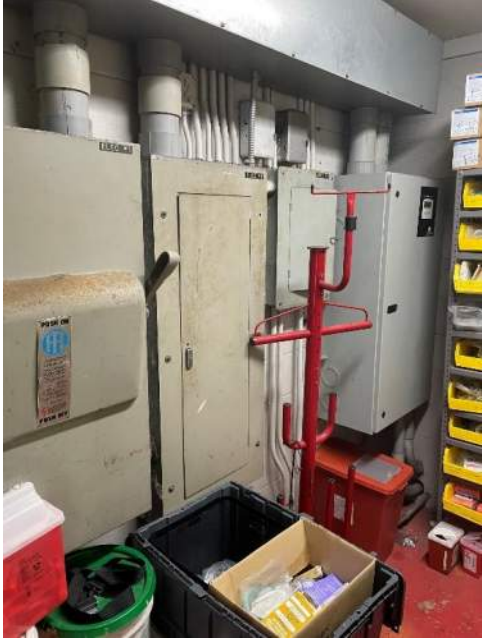
IMG_4262: Electrical room main disconnect, MDP, Panel A and ATS
