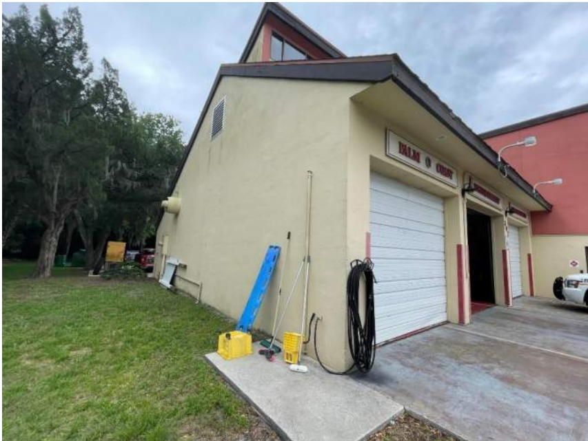
IMG_7886: Apparatus bay exhaust fan discharging to louver in east wall
