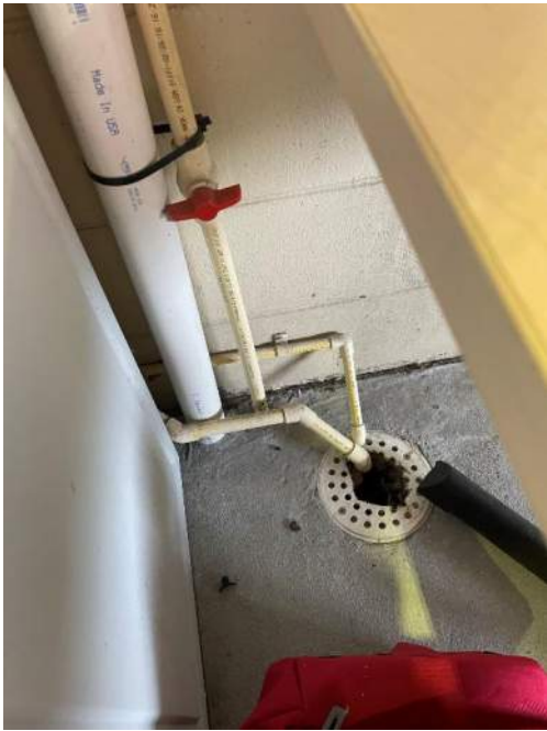
IMG_4467: Floor Drain needs replacement.
