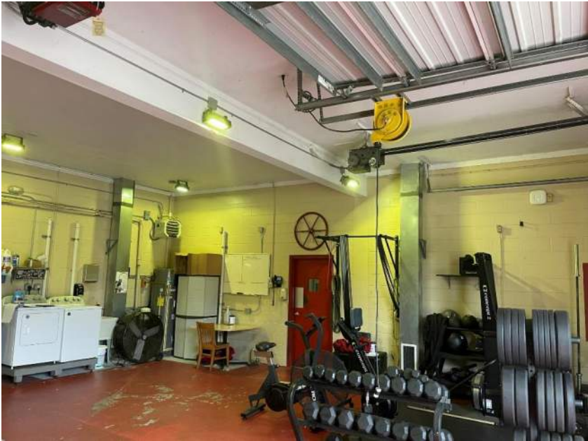
IMG_4288: Apparatus Bay LED floodlights
