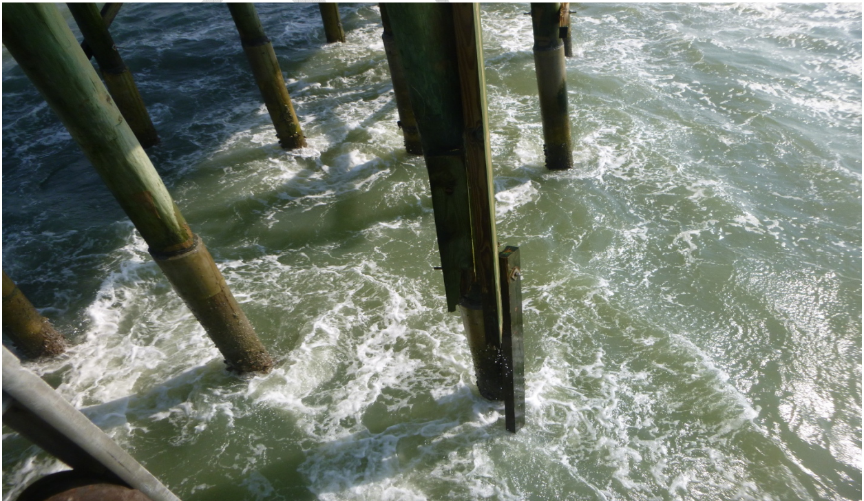
BENT 17 TO 18 FAILED CROSS BRACING
