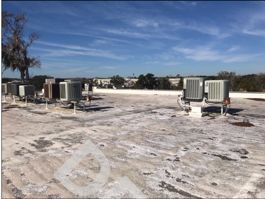
11 - HVAC units on the roof of the three-story office building.
