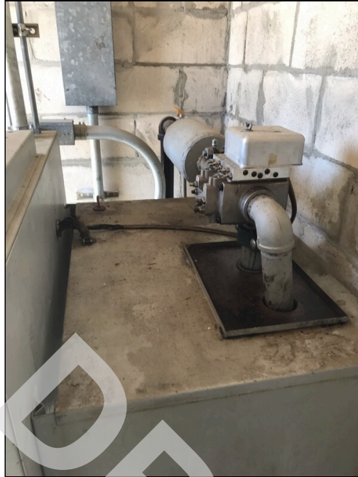
15 - Hydraulic oil reservoir in the elevator maintenance room on the roof.
