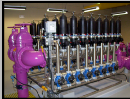
1 Effluent Pumping Facility
