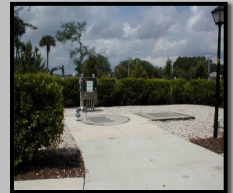
165 Wastewater Pump Stations
