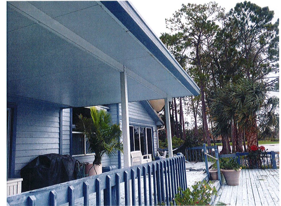
After Hurricane Irma
