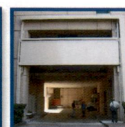
Vertical Lift Flood Barrier
